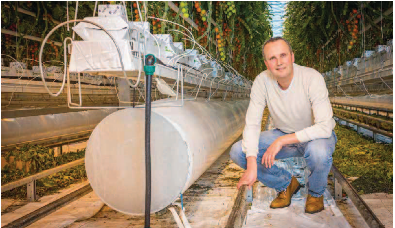
According to Jeroen Steenbrink, the central heating element in the system plays a key role as it prevents very cold air being brought in at the bottom of the greenhouse.”
